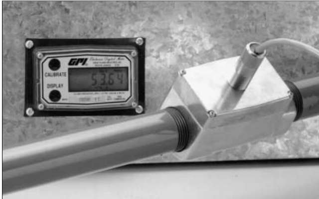
Remote Kit installed with GPI Electronic Digital Meter.
